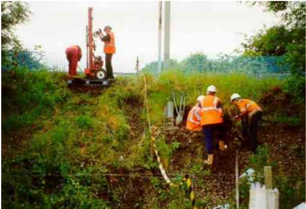
Figure 8. – Dynamic Probing, Window Sampling and Hand Pitting in use on a railway embankment
